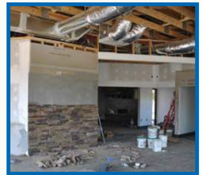
Specialty features such as brick are incorporated in restaurant design.
